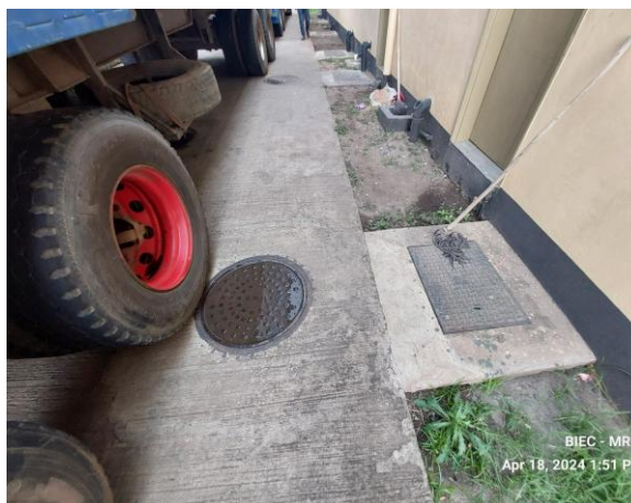
Figure 4-10. Septic tanks at the site
