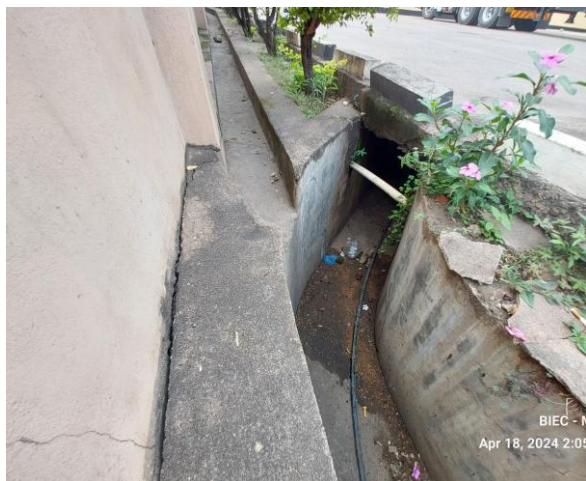
Figure 4-2. Open drain taking water out of the BIEC facility.
